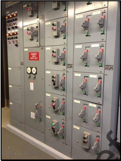
Wastewater Treatment Plant
