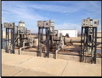
Wastewater Treatment Plant
